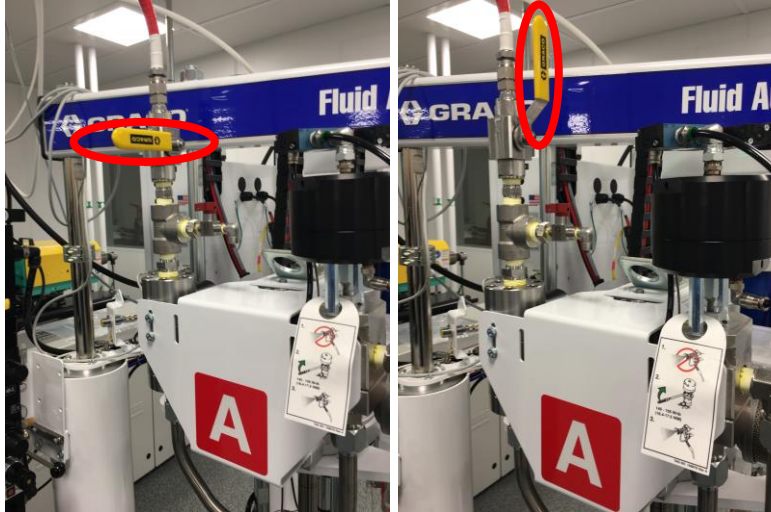
OFF position (horizontal) ON position (vertical)
