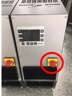
Main power switch in the OFF position.
