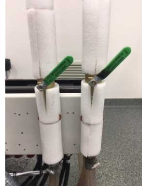
Valves in the ON Position
